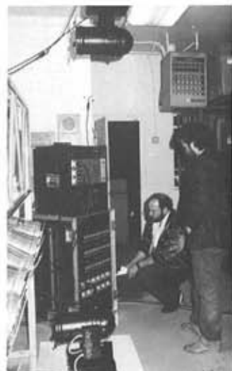
Mark Ward (right) of Celco Inc. discusses Celco's new dimmer system with Brian Gale, consultant to Disneyland.
